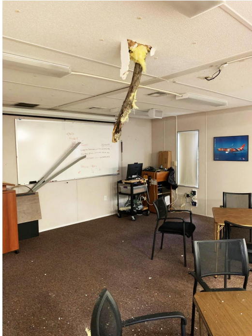
Limb Damage to TA-2 Classroom at Tallwood, September 12 (No Harm to Personnel or Equipment); It Is Under Repair by Mason Facilities
